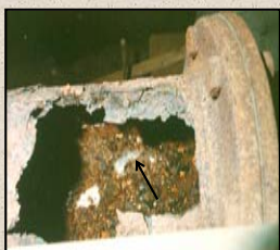
Hg found in pipelines and building structures
